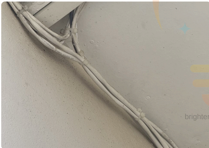
Conductor bundles routed around the home. Every power-injection point adds more wire to hide — and more places to fail.
