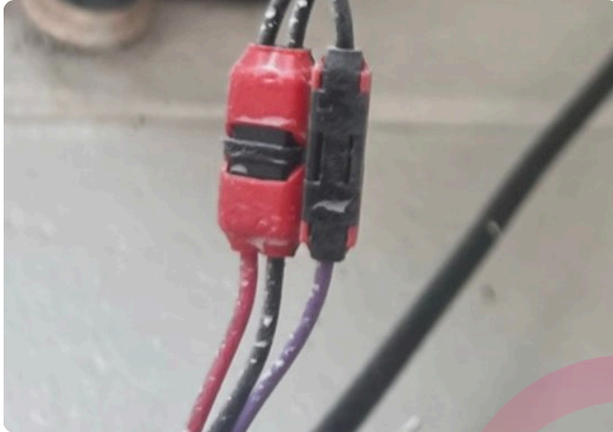
Field splices at the roofline. Tap connectors joining cut conductors, exposed to heat, moisture, and movement. Multiply this by roughly a hundred per job.
