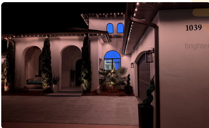
Detail at the eave. Fixtures sit recessed in the color-matched channel; the beam is aimed down and back at the wall.
